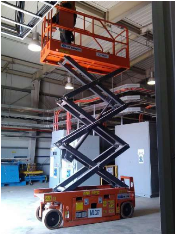
GTJZ0608 for facility maintenance
